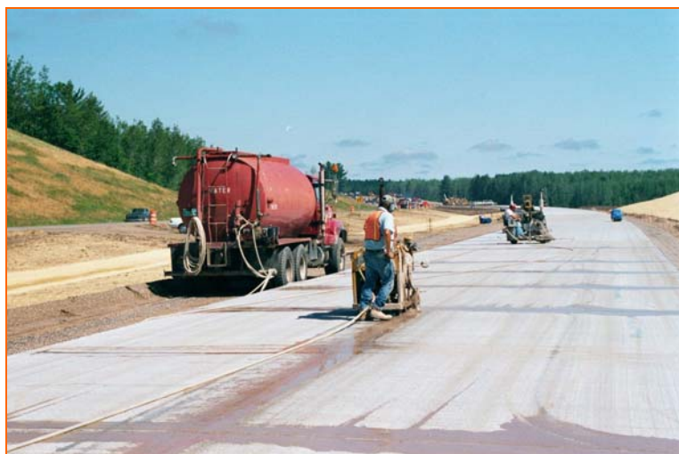
Control joints should be cut as soon as possible to control crack potential
